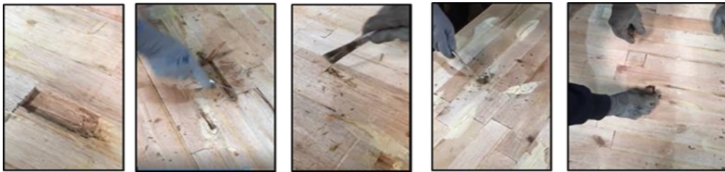
Figure 1. Picture of product defect
